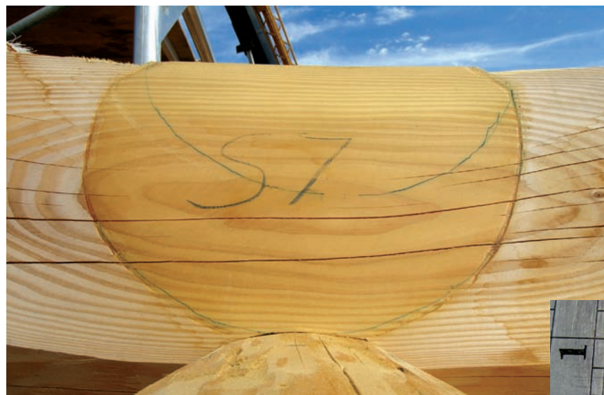
Figure 6.b: In the building yard, about 100% of the weight of the building is on the notches, and very little weight is on the grooves. In this photo you can see that the notch has compressed the saddle, and this is the result that we want.
