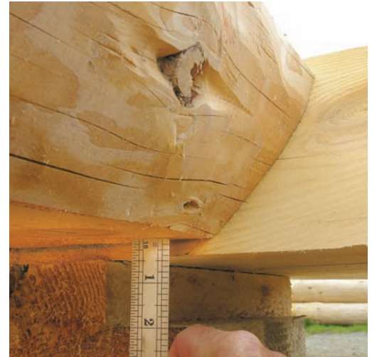
Figure 6.a: Sill logs, showing the underscribe amount. For sill logs, the difference in height between the three-quarter-sill-log flat and the half-sill-log flat is the underscribe amount.
